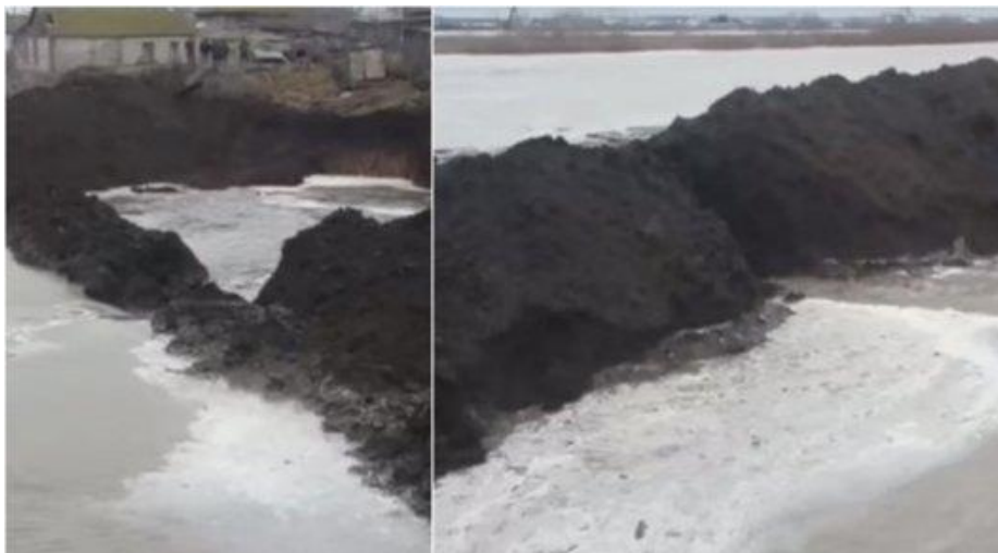
Figure 6.51. Destruction of the embankment dam near the town of Atbasar in 2017 https://tengrinews.kz/kazakhstan_news/pavodki-v-kazahstane-live-316268/
